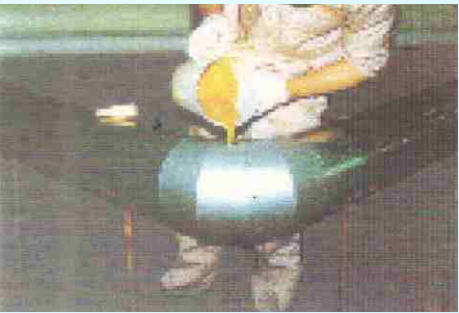
Pour Chemicals through opening
